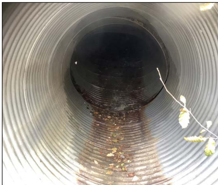
Photo 3. Facing upstream showing damaged culvert
