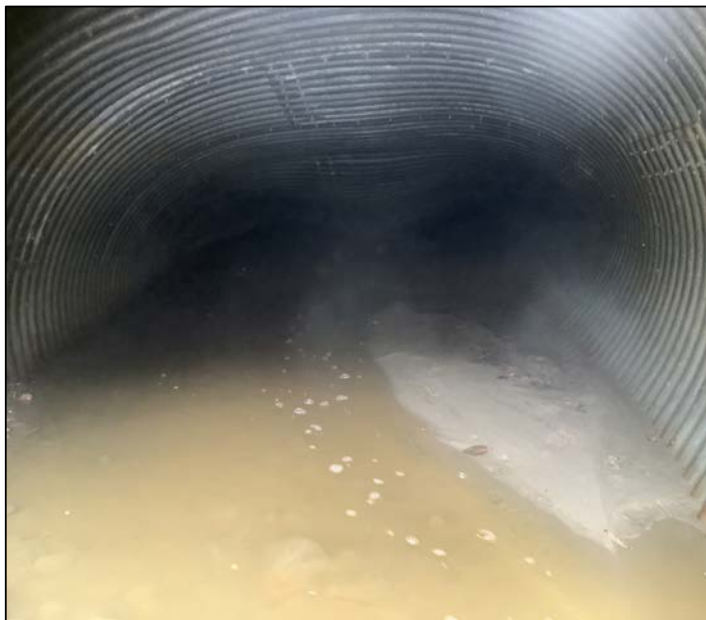
Photo 1. Facing outlet, culvert collapsed in centre
